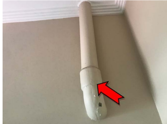
Photo 2. Interior, ground level, staff toilet adjacent to staffroom, down pipe – asbestos-containing moulded fibre cement.
