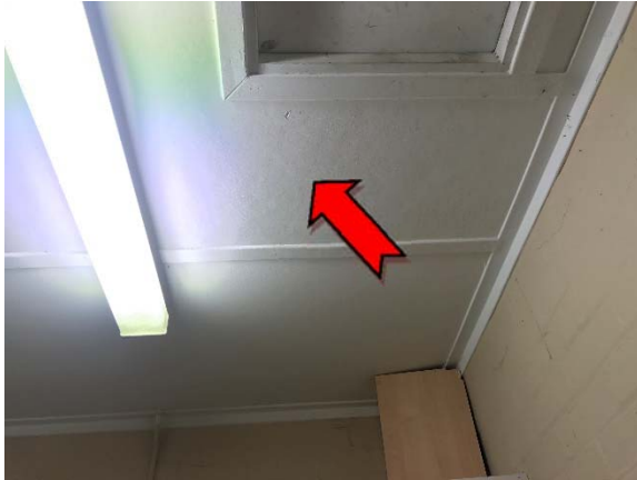
Photo 1. Interior, ground level, laundry room, ceiling – asbestos-containing fibre cement sheeting
